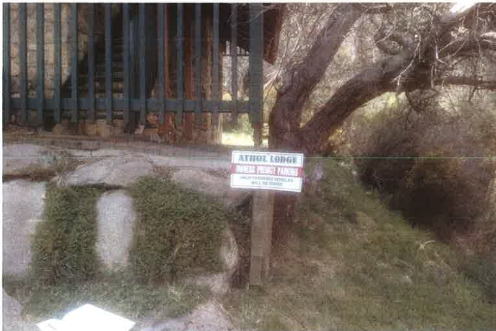
Photo 4 – View of existing retaining wall and awning posts along the western side of site
